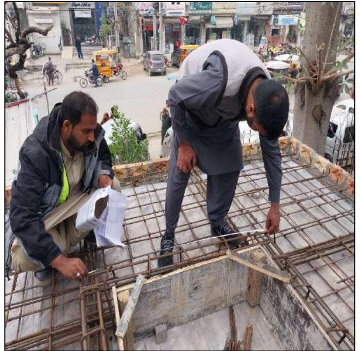
Picture 60: Steel Fixing of Roof slab of Pump Room at Civil Hospital
