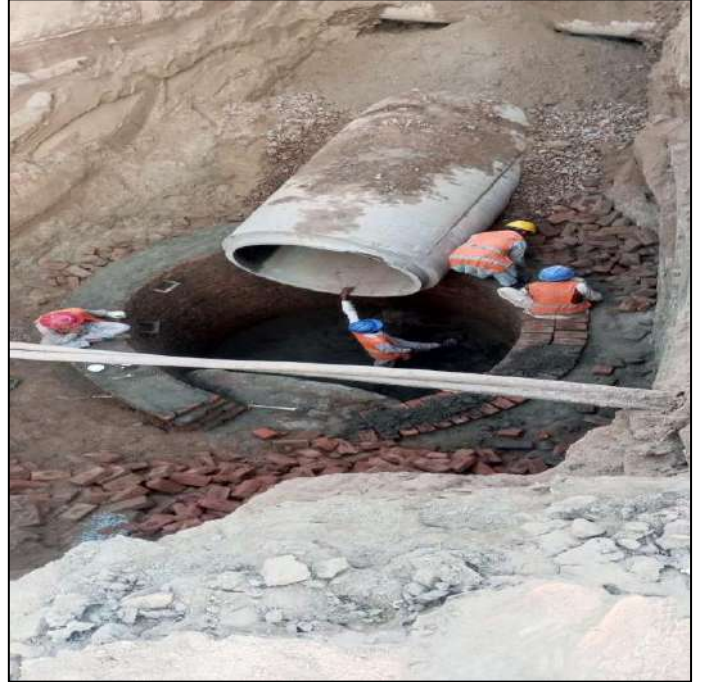
Picture 24: Construction of manholes at 54" dia & 60" dia L-1 (Arratulla Road) in progress
