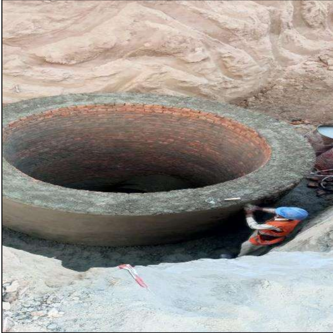
Picture 23: Construction of manholes at 54" dia & 60" dia L-1 (Arratulla Road) in progress
